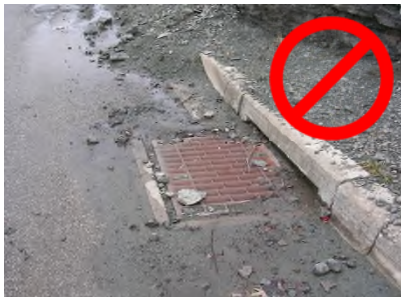
Protect storm drains – keep muddy and polluted runoff out.
