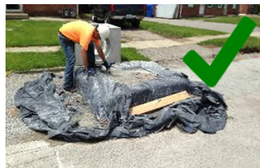
Cover wastes and materials that might leach pollutants.
