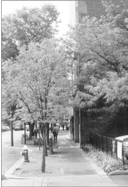
Sidewalks vary in construction and quality in the area.
