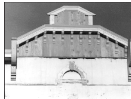
Reconstructing missing details, when sufficient information is available, is encouraged. In this case, the original cornice is missing in the photo at upper left. The central portion of the pediment is under construction, above. When completed, in the photo at lower left, the shadow lines from the cornice once again add interest to the building front.
