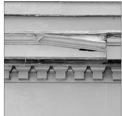
Repair those features that are damaged.
